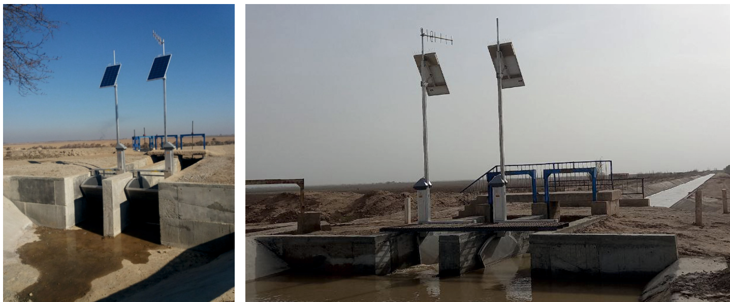
Figure 5. The Mirishkor-Kamashi Canal automated by Rubikon Water Pty. Ltd.
